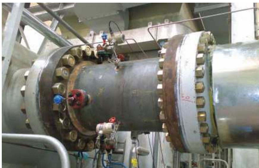
■ Figure 3. Temporary instrumentation installed on a centrifugal compressor suction line.
